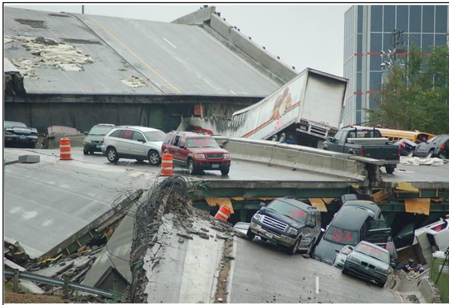
Fig. 1: Bridge collapse, Minneapolis, MN, Sept 2007
